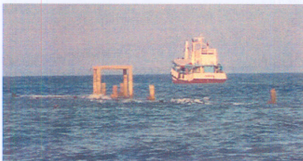
Bengali Jetty damaged and submerged under sea water at Teressa
