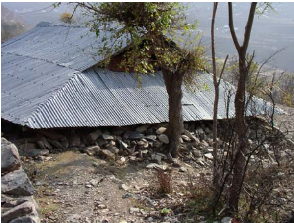
Photo. 9:- Salamabad House – Collapsed Uncoursed Random Masonry with intact roof.
