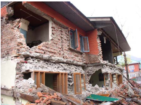
Photo. 1:- Uri town – Police Station – Delamination & collapse of Burnt Brick Cement Masonry walls and Un Coursed Random Cement walls
