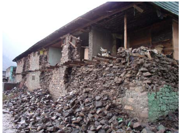
Photo. 2:- Uri town – Shops – Delamination of Un Coursed Random in Mud Masonry wall with Corrugated Galvanised Iron roof.
