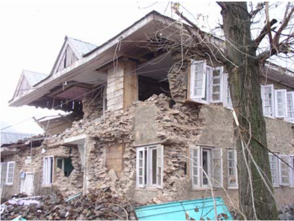
Photo. 3:- Uri town – Govt. Quaters – Delamination & collapse of Uncoursed Random Masonry walls (no ‘through’ stones) with intact Corrugated Galvanised Iron roof.
