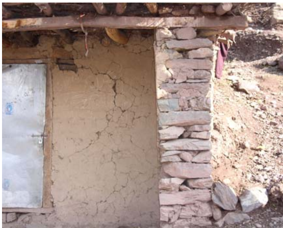
Photo. 5:- Uri town – Shops –Collapse of Uncoursed Random Mud Masonry walls with Reinforced Cement Concrete slab.
