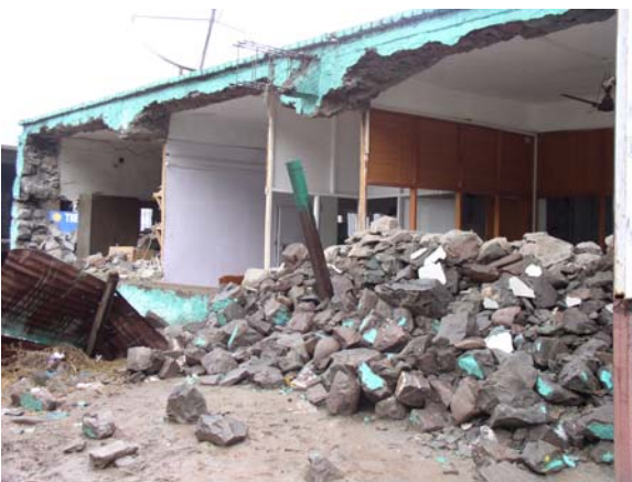
Photo. 7:- Near Sultan Gaddi – House - Uncoursed Random Masonry wall with ‘through’ and long stones (saved from collapse).
