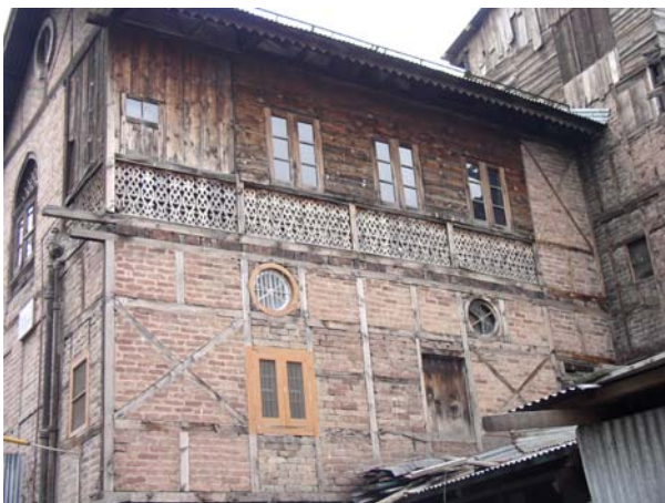
Photo.11:- Srinagar – Combination of Dhajji type & wooden wall (More diagonal braces needed).
