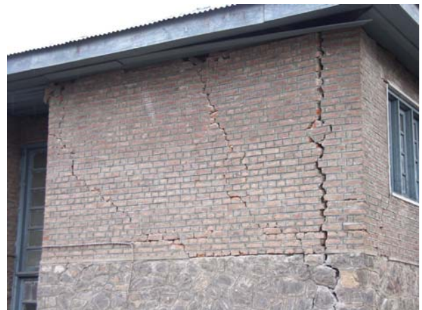
Photo.6:- Uri town – Civil Defence Bldg.– Corner cracks and vertical cracks in Burnt Brick Cement Masonry wall.
