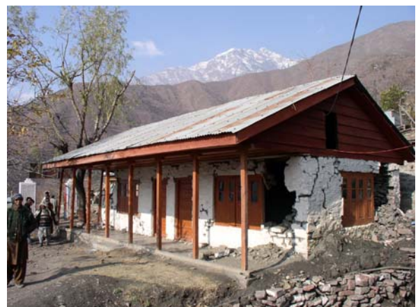
Photo. 8:- Sultan Gaddi – School – Collapse & cracking of Uncoursed Random Cement Masonry walls with intact roof (walls can be rebuilt with safety features).
