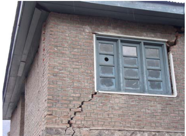
Photo. 4:- Uri town – Civil Defence Bldg.– Diagonal cracks in window openings and tilting of walls in Burnt Brick Cement Masonry wall.
