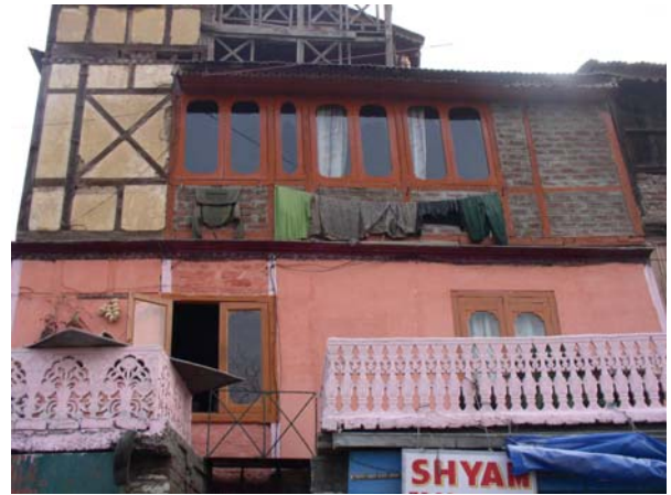
Photo.10:- Srinagar – Dhajji type of wall – Old & new ( more diagonal braces needed).
