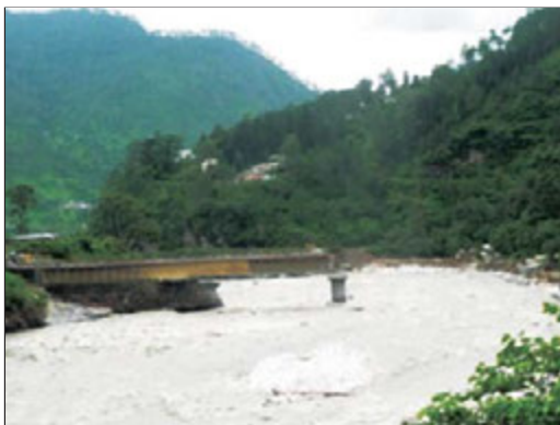
Fig.4.61: Damaged support works of the Gangori bridge after flashfloods in Asi Ganga Valley
