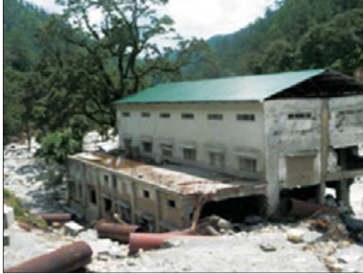
Fig.4.33: Power house gets damaged and filled with river debris during flashfloods in Asi Ganga River
