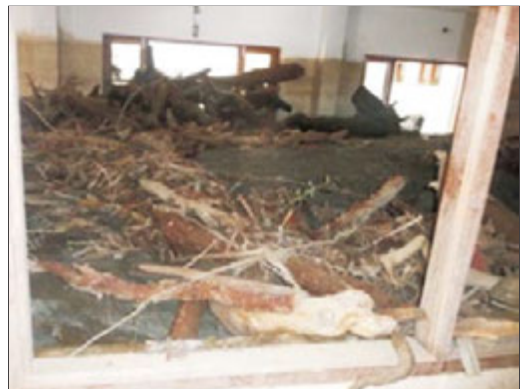
Fig.4.6: The building got filled with river debris upto the lintel level above windows near Asi Ganga River at Gangori
