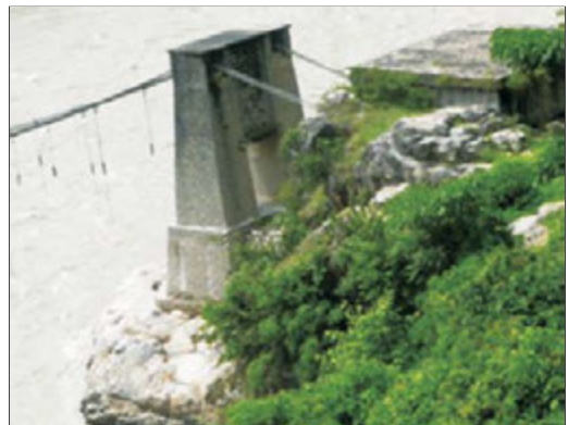
Fig.4.54: The tower on rock beds still exists while the tower on the other side of suspension bridge washed away by flashfloods
