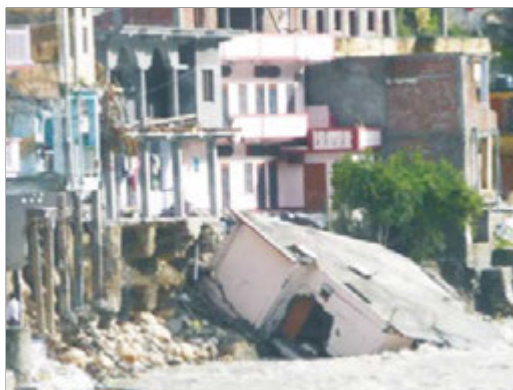
Fig.4.19: Completely collapsed building falls in the river
