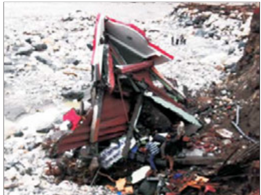
Fig.4.12: Complete collapse of bank building situated near Asi Ganga River at Gangori
