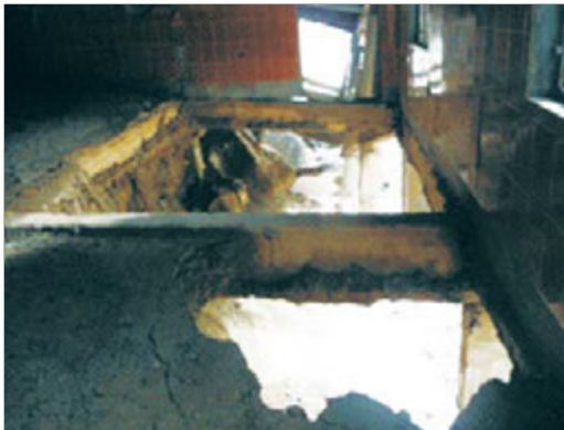
Fig.4.29: Foundation and floor of the building eroded completely by flashfloods
