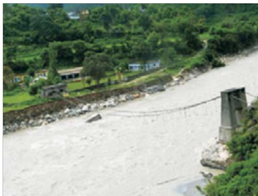
Fig.4.55: A view of the suspension bridge whose one pier / towers were damaged during flashfloods
