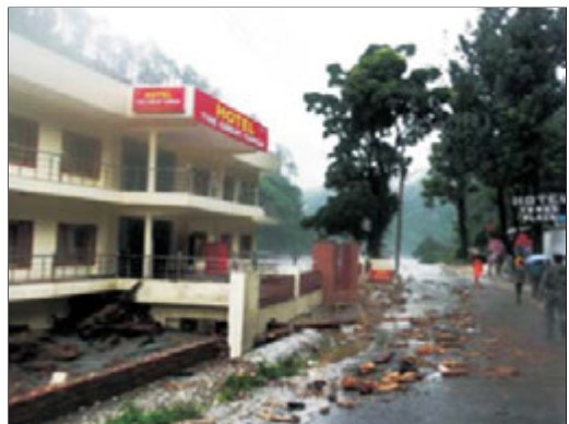
Fig.4.14: Front view of the hotel building affected by the flash flood debris
