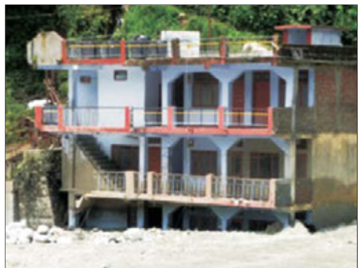
Fig.4.26: River water fills the ground floor of a building situated near Asi Ganga River at Gangori
