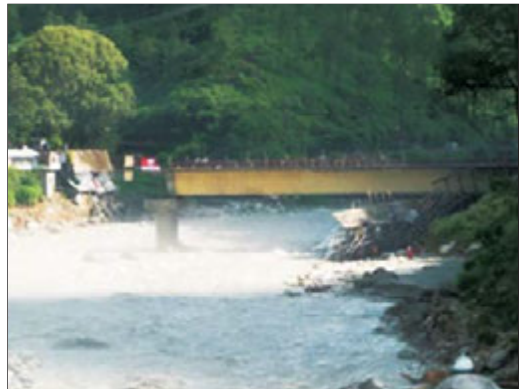
Fig.4.60: Support works for bridge construction got badly damaged at Gangori after the flashfloods
