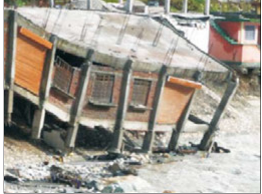
Fig.4.34: Erosion of foundation leads to columnar failure and collapse of a new building after the flashfloods
