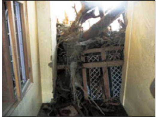
Fig.4.10: River debris damages and blocks the way in the hotel building situated near Asi Ganga River at Gangori
