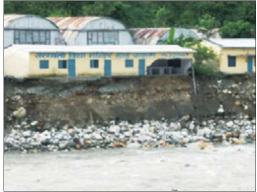
Fig.4.22: School building endangered after erosion of river banks and partially damaged foundations
