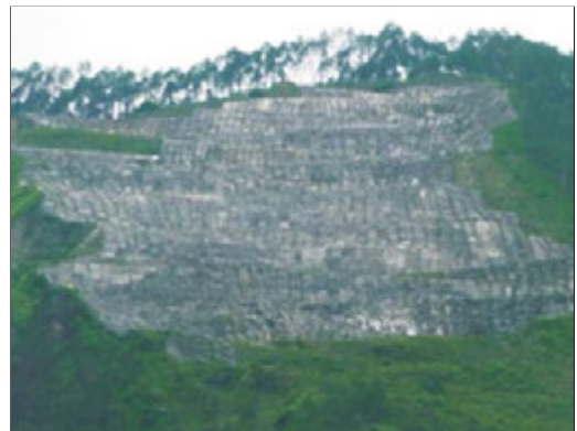
Fig.4.48: Huge treatment works at the headscarps of Varunawat landslide tends to reduce the problem
