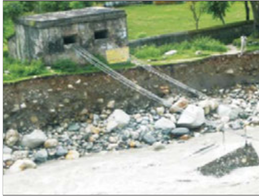
Fig.4.51: The tower of a suspension bridge fails after flashflood in Uttarkashi
