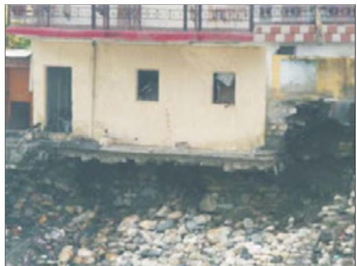
Fig.4.62: Building Foundations on the riverside were eroded and damaged after flashfloods, leaving it unusable
