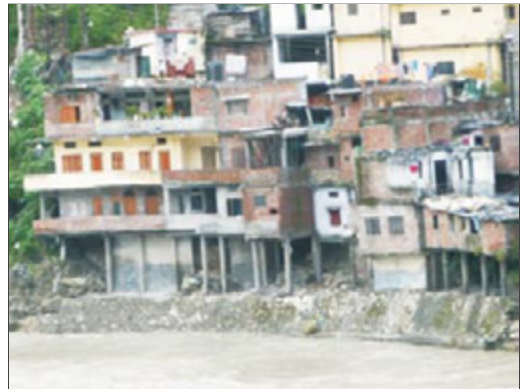
Fig.4.30: Insufficient Embankment protection works for safety of building close to river
