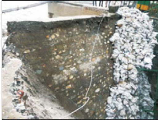
Fig.4.39: Protection provided by sand bags at Tiloth Bridge
