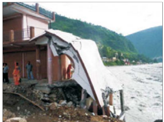
Fig.4.32: Frontal part of the building completely collapsed after the flashfloods in Bhagirathi river
