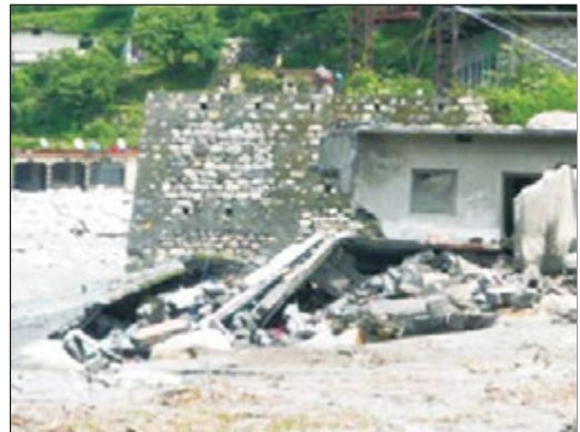
Fig.5.28: Collapsed building situated near Asi Ganga River at Gangori
