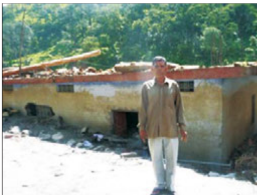
Fig.4.13: Victim who lost his house (in the background). River sediments and tree logs damaged building and over-rided building and over-rided roof
