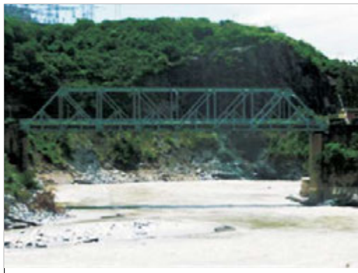
Fig.4.53: Narrow section and placement of piers on or close to river poses danger of its being washed away during flashfloods
