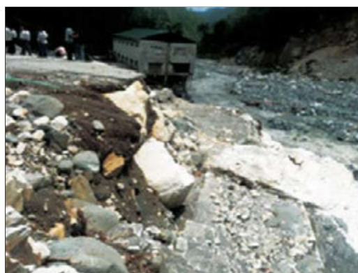
Fig.4.66: A hotel building on the verge of collapse due to damages to foundation after the flashfloods in Asi Ganga Valley
