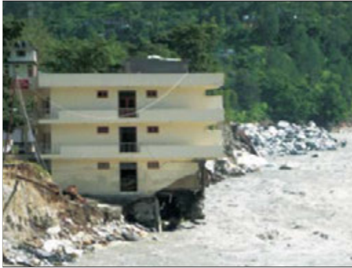
Fig.4.3: A hotel building lost its foundation during flashfloods in Asi Ganga River
