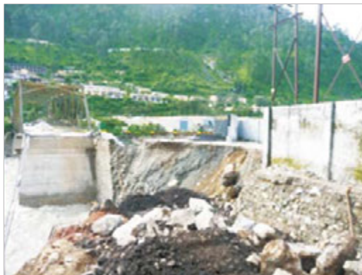
Fig.4.17: Link road to the bridge at Tiloth destroyed by flashfloods in Bhagirathi river
