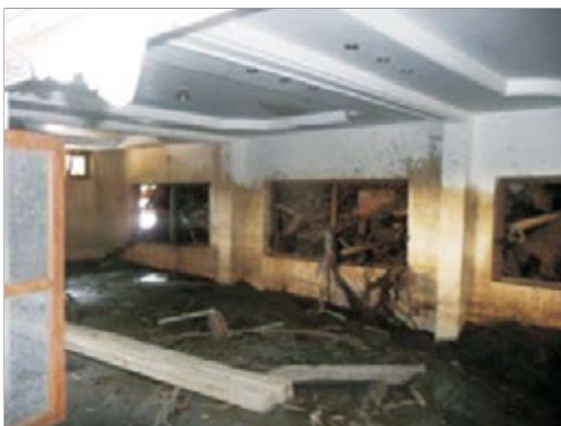
Fig.4.7: Hotel building completely choked with river debris after flashfloods in Asi Ganga River at Gangori
