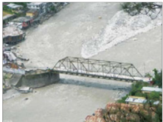
Fig.4.56: Such location where the river section suddenly narrows down are susceptible to erosion during flashfloods
