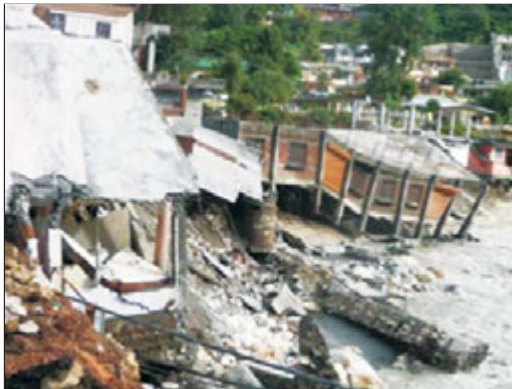
Fig.4.23: Embankment walls and building foundations eroded after flashfloods cause structural collapse
