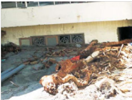
Fig.4.5: Debris entered behind the rooms on riverside and choked the way
