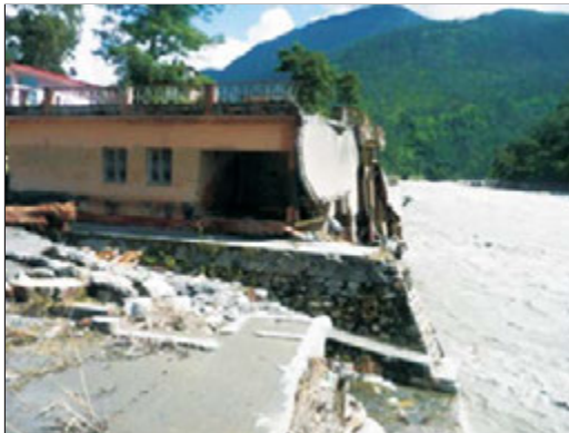
Fig.4.11: Roof collapse and debris accumulation on the top of a house at Gangori
