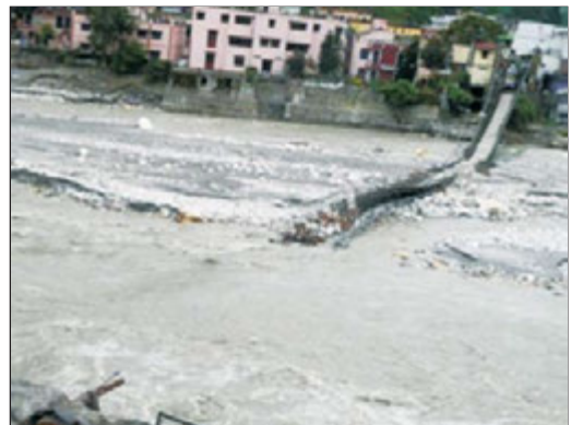
Fig.5.30: Suspension bridge in Uttarkashi was detached after its pier/tower got damaged by flashfloods
