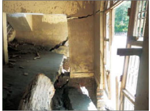
Fig.4.16: A Collapsed building on riverside after the flashfloods in Asi Ganga
