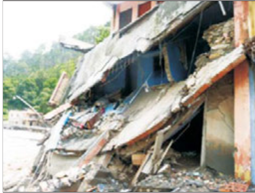
Fig.4.15: Complete collapse of building near Asi Ganga River at Gangori
