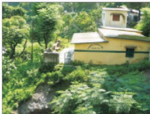
Fig.4.64: A primary school building located at the crown of a landslide poses an impending risk at Khari
