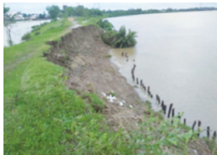
Figure 5.3: Damage of Keradagada Altnaga saline Embankment on Hansua right due to Cyclone “YAAS”. (Source: Government of Odisha Memorandum on Very Severe Cyclonic Storm, Yaas, May 2021)
