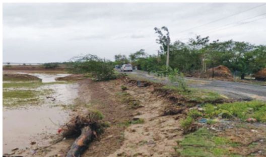
Figure 5.2: Damage of Naliatapatia Talachua Saline Embankment due to “YAAS.” (Source: Government of Odisha Memorandum on Very Severe Cyclonic Storm, Yaas, May 2021)
