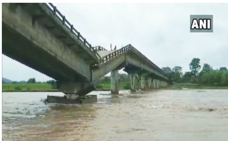
Figure 3.14: A Collapsed Bridge in Ranchi. (Source: Times of India)
