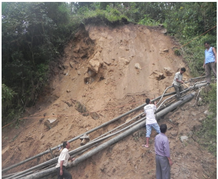
Fig. g-4. Landslides caused severe trouble to dwindling infrastructures services and utilities. Once again restoration of the same has hardly any technology in place
