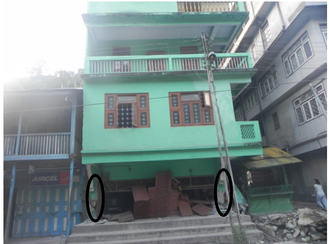
Fig. e-2.. This pvt. Building at Singtam town lost load bearing power to two of the front columns at ground floor, thus it could be a fit case for demolition. However, it was found that this building suffered very little structural damage to the upper floors. The amount required for proper retrofitting of the same could be much less than demolition and thereby fresh construction cost by the owner. The govt. need to devise proper policy for load sharing of reconstruction burden else punitive order to carryout such work by affected owner would be difficult to sustain.
