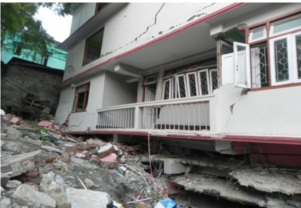
Sikkim collapsed during earthquake. This has to be demolished completely
