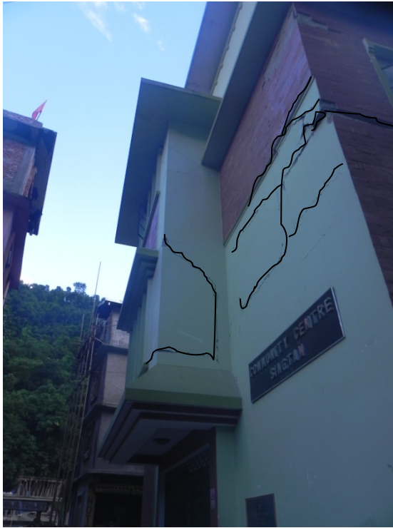
Fig. e-1. Cracks in Community Centre, Singtam and many such buildings can be repaired and retrofitted without much cost and time . Just deciding to demolish these kinds of buildings without detail structural safety assessment would be rather unwise and costly exercise.
