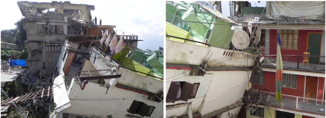
Fig. d-1. Two buildings at Baluakhani developed excessive tilt on 23 rd Sept 2011. Special team from Hyderabad were engaged for demolition. Several buildings in Gangtok have been declared unfit and they are being demolished one by one. However, it important to look into the safety of these buildings by expert team. It would be wise to check if retrofitting is possible by careful planning and supervision of the entire works. Some guidelines for damage survey are given in the appendix.
