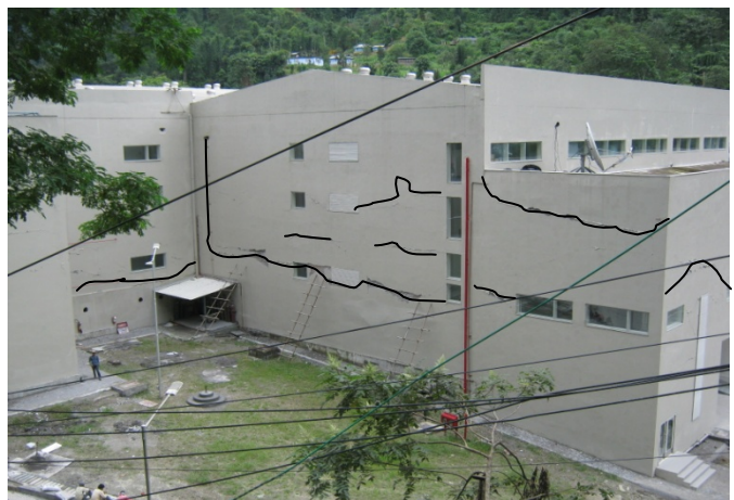
Fig. e-4. Torrent Pharmaceutical Industry complex, with more than 500 employees, near Sikkim Supreme Factory, NH31A, suffered severe damage in the walls. Upon inspection of the same it was conveyed that owner shall be taking sufficient measures to restore everything. It is required to have a check on such commitments by pvt. Industries and hydroelectric project authorities.
