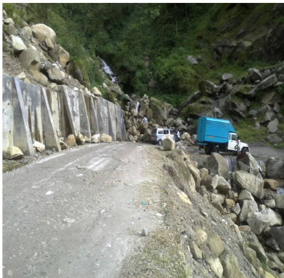
Fig. g-3. Controlling measures around the Bagthang water falls, in the form of buttressed retaining walls are no way effective in preventing landslides. The road has no culvert or x-drains. Boulders are constant threat to unwary travellers.
