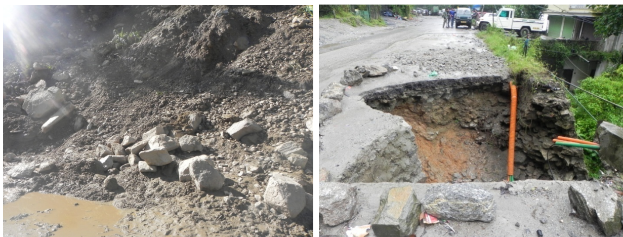
Figure 17 Landslides along NH31A. earthquake has triggered several landslides along national highways. The fragility of roads in the hilly area has been exposed by this earthquake, which otherwise too vulnerable to season rain fall. Road widening works in many roads has made them more vulnerable than before. BRO has been active in removing debris but not yet so effective on the promulgation of new technologies. Clearing roads just for allowing one way traffic for the time being is not enough to continue with the ongoing power house construction project. Teesta stage III project is now on halt due to labour shortage. They fled after the earthquake.
