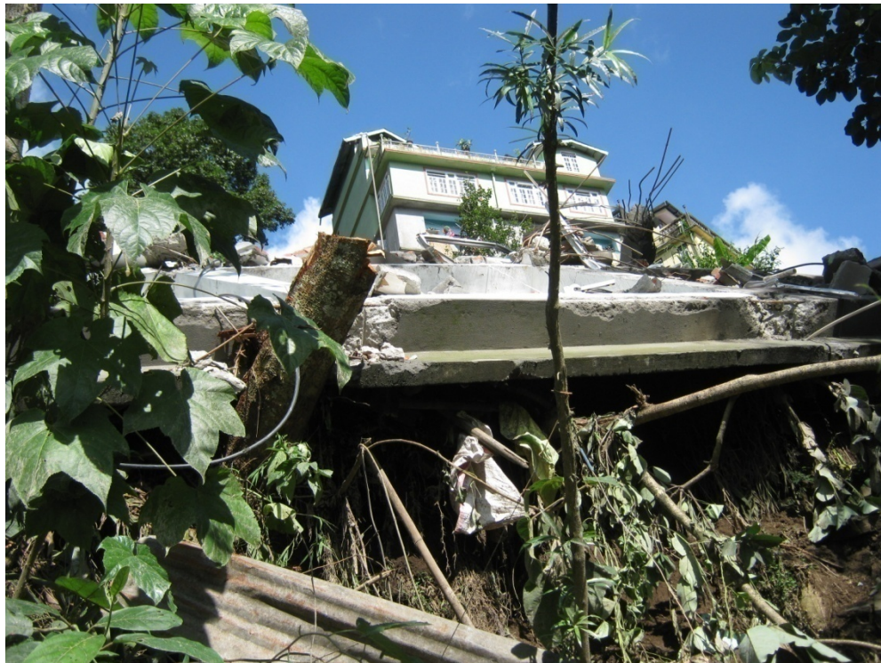
Figure 11 One 3 storey newly constructed building near Lumsey primary school, Gangtok collapsed during earthquake. Reason for failure not known yet. Approach road for demolition equipments are not available. Debris are precariously retained till date by few trees, main trunk of which were cut by electric power department
