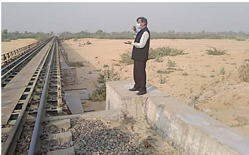
Figure 28: Sand deposit in Rel River at Gogabapaji Railway Overbridge, Dhanera (Picture captured on 4/01/2021)
