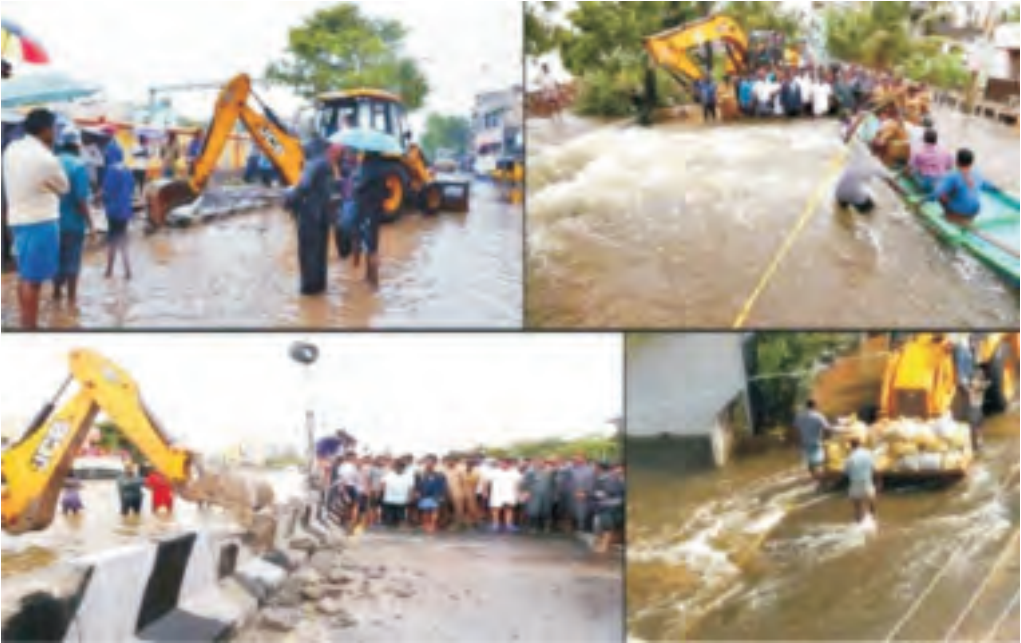
Figure 5.7: Clearance of Flood Water and debris by the Government Authorities Source: (GCC, 2017)
