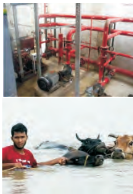
Figure 5.5: Damaged MEP systems and cattle stuck in floods(left to right) Source: AIR; WordPress
