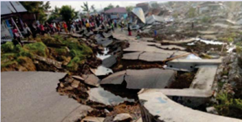
Figure D-4: Picture Depicting the Extent of Damage due to Earthquake in Yogyakarta
